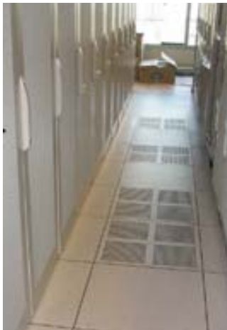
Figure 2B: Hot aisle
